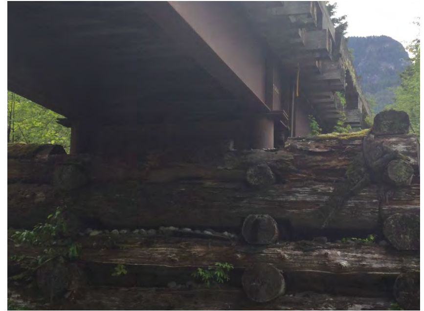
Top log condition on right side of pier
