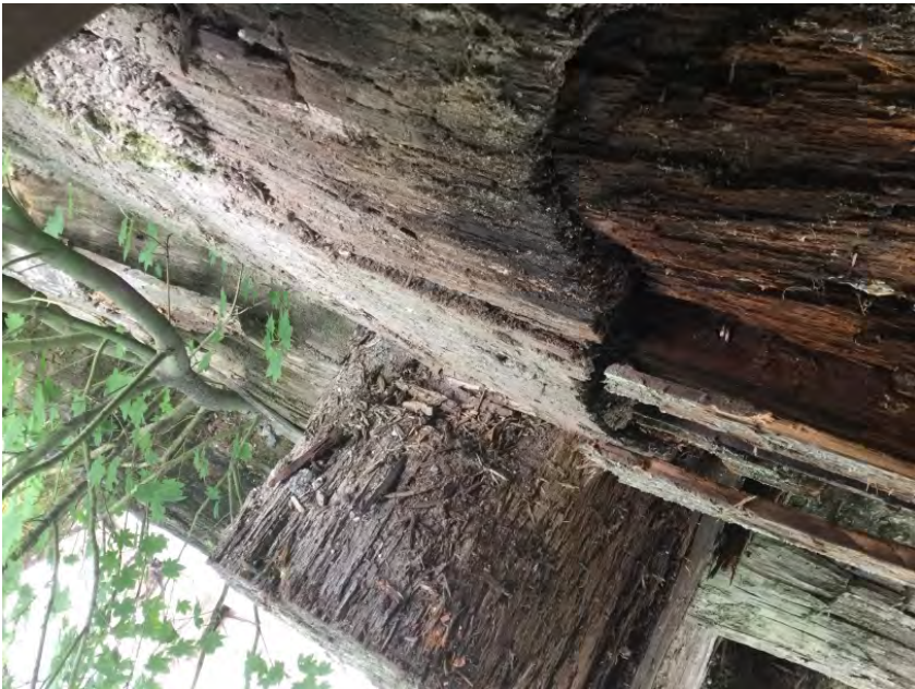
Poor condition of top crib log at downstream left side of pier
