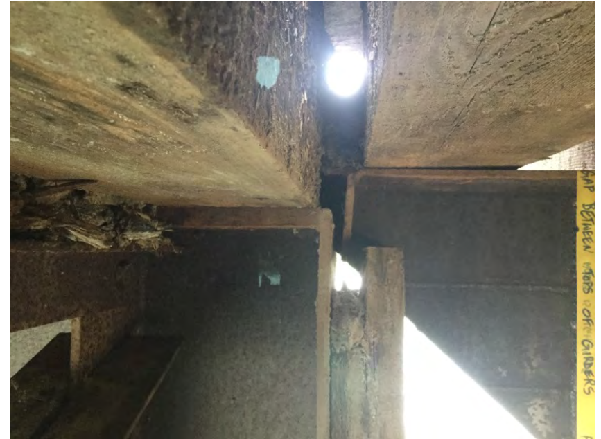
Left span girder 55mm lower than right span at downstream location
