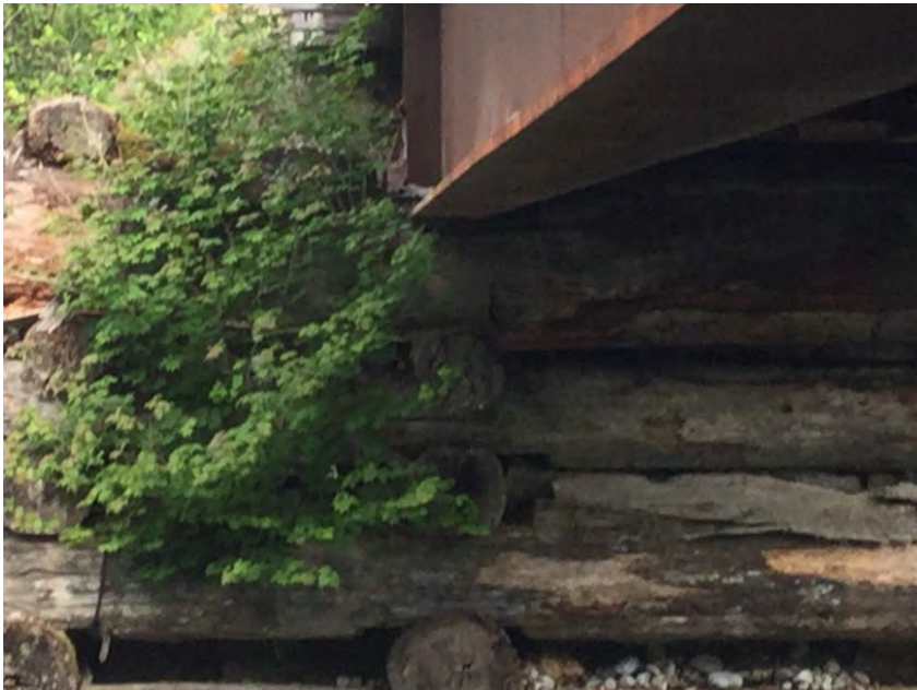
Top crib log on left side of pier in poor condition and downstream left span girder 55mm lower than right span
